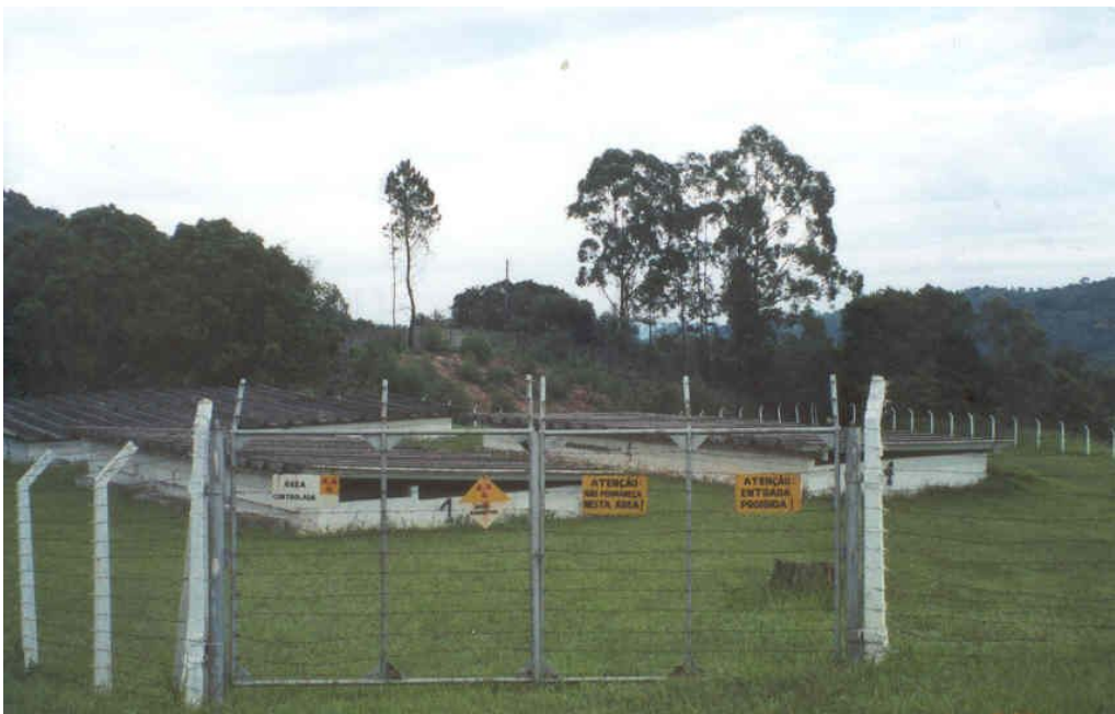
Figure 2: Storage Concrete Pools
