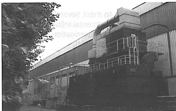
Flue gas purification
