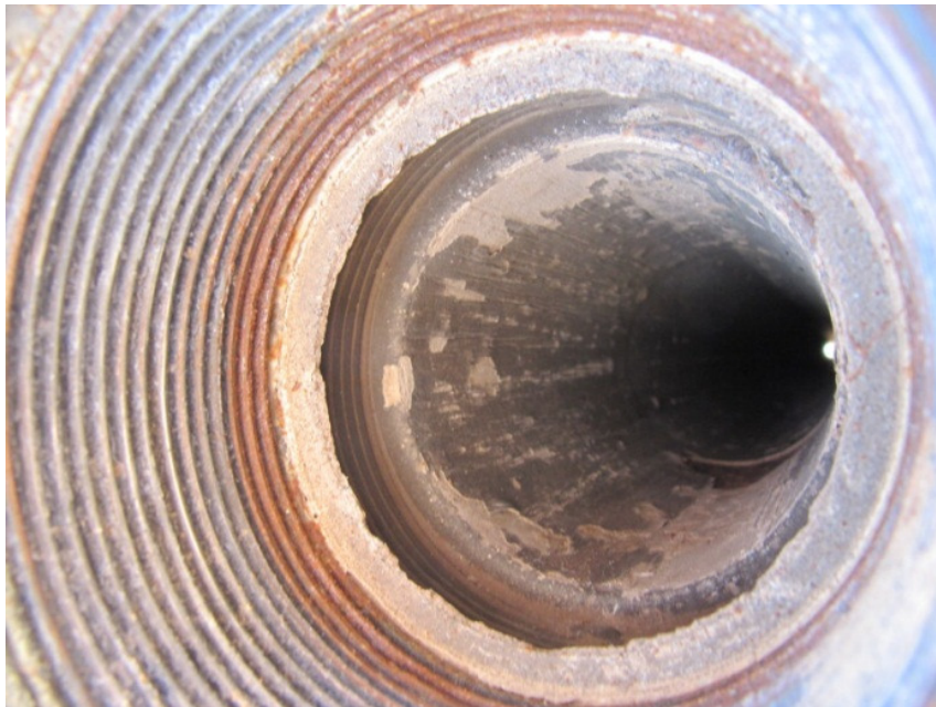
Contaminated Tube Pre decontamination
