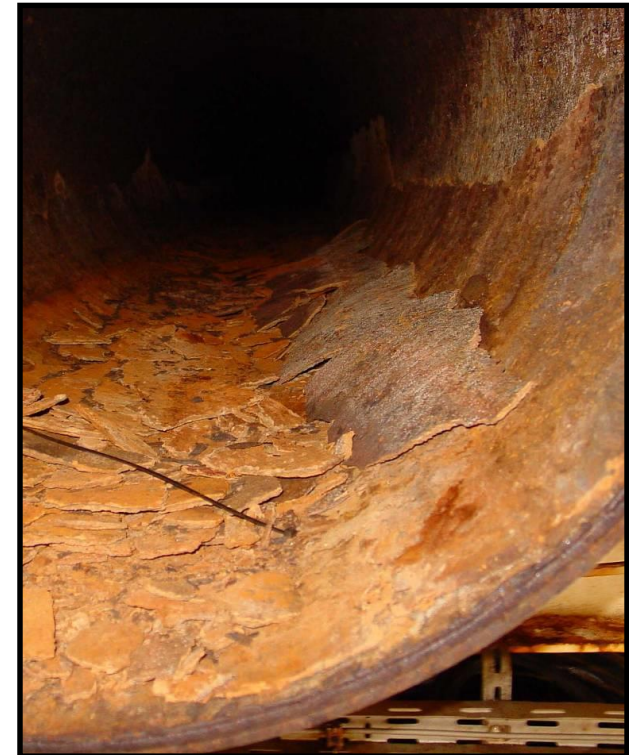
Ba sulphate Scale in oil export pipe.
